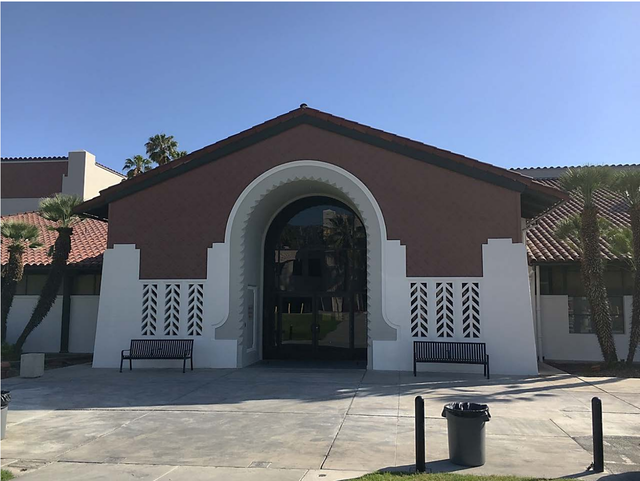
Figure 11: Glendale Civic Auditorium, detail of entrance bay, main façade, view south of entrance after 1963 entrance loggia was removed. Exterior paint scheme was changed as shown in early 2017. Compare to photograph in Figure 12. May 2017, TGHS.
